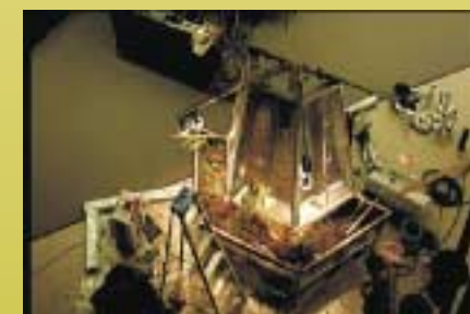
The new biofilter being constructed at NORCAT (Northern Centre for Advanced Technology) in Sudbury Ontario. This biofilter was commissioned with northern Boreal species.
